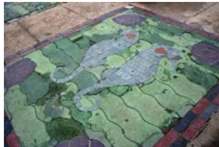
Detail of one of three panels that comprise the Central Mall mosaics showing general deteriorated conditions, 2010.
